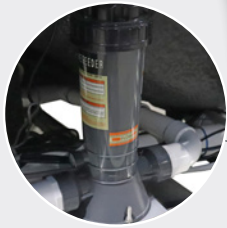
In-line dosing system hidden within the cabinet
